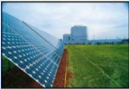
DTE solar array in Southfield, MI
